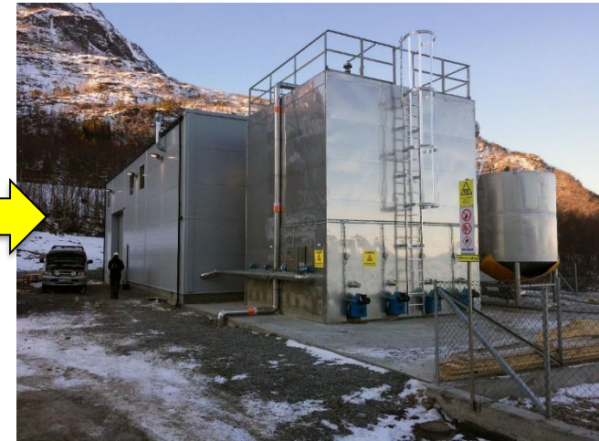
100 m 3 anaerobic baffled bioreactor
