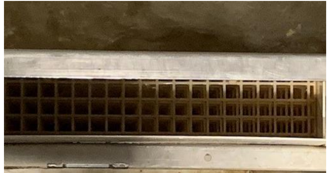
Degasser in use at Vikan Settefisk Zero biofouling In use ca 3 months
